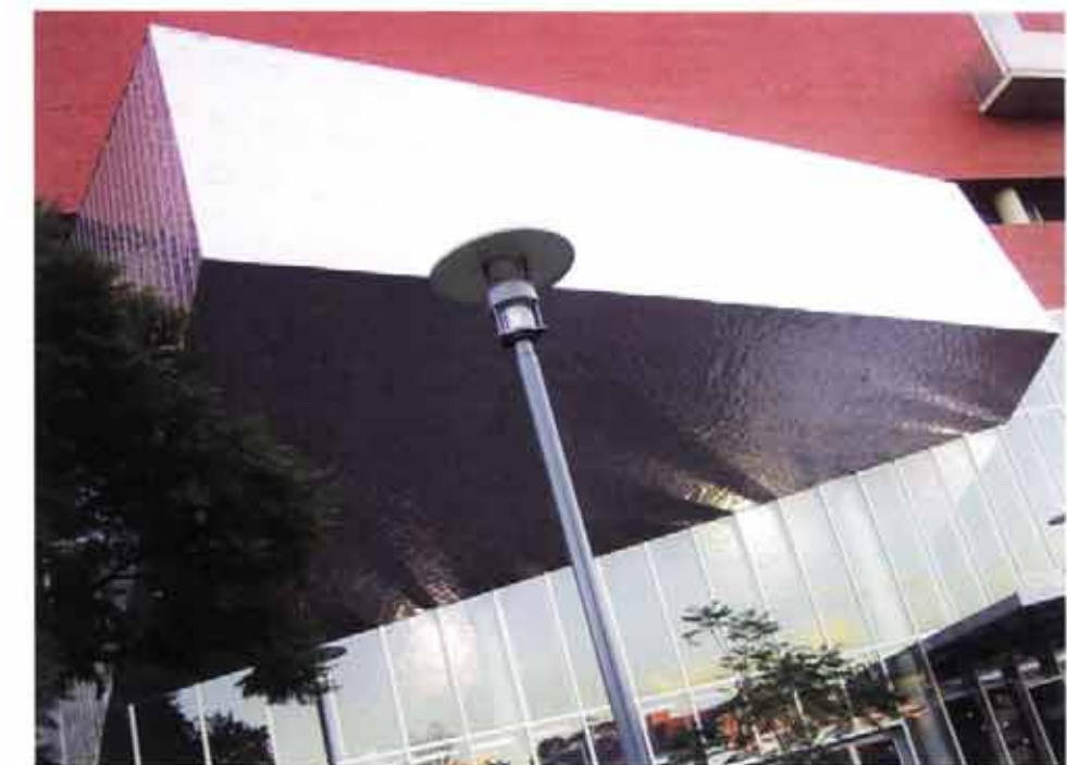
ABOVE: A successful stainless steel installation in an outdoor application.
